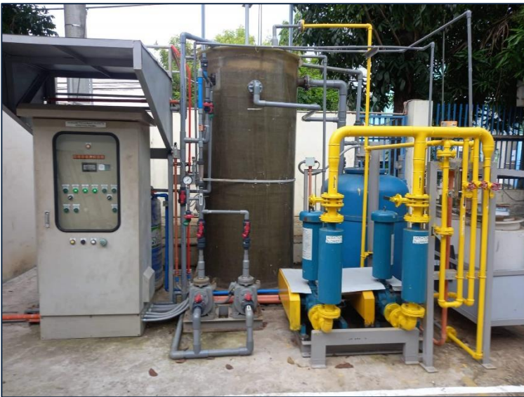
Sewage Treatment Plant 2 Philippines Ogami Corporation Using MBR Technology 1.5m 3 /Day
